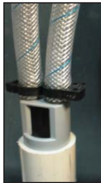
S. Drain hoses connected to air gap at drain pipe
